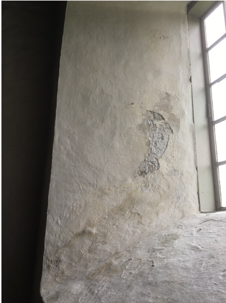
Image 8 Damages from salt crystallization inside Skoger old church In Buskerud, Norway. Photo: NIKU
