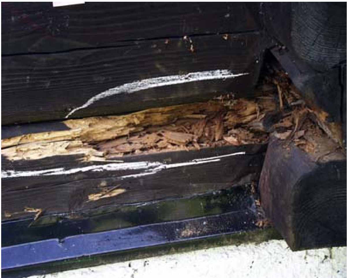
Image 2 Rot damages. Often, the inner parts of the logs are attacked, while the surface is relatively intact. Photo: Mycoteam
