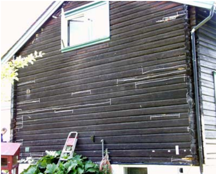
Image 3 Mapping of rot damages in a timber wall. Photo: Mycoteam
