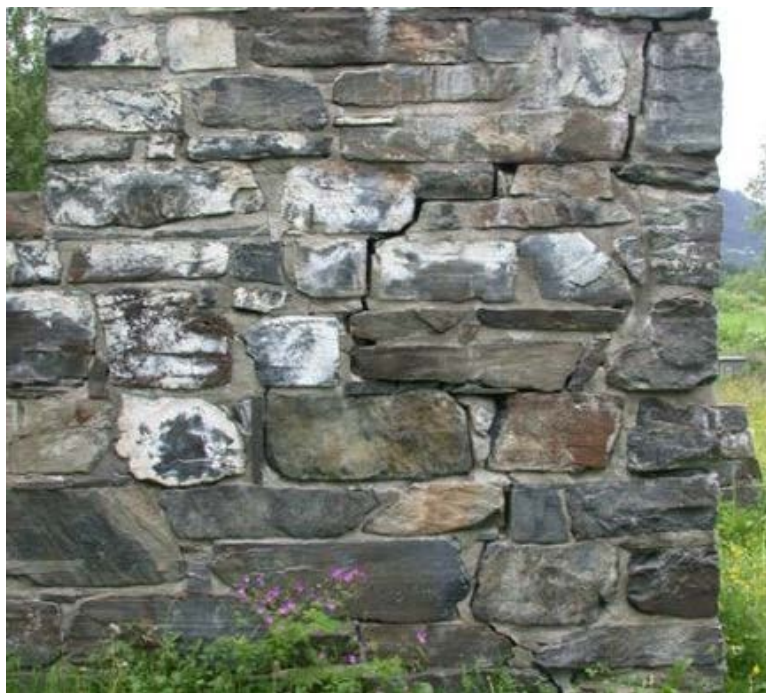
Image 7 Frost damaged masonry at Mo church ruin, Valdres, Norway. Photo: NIKU
