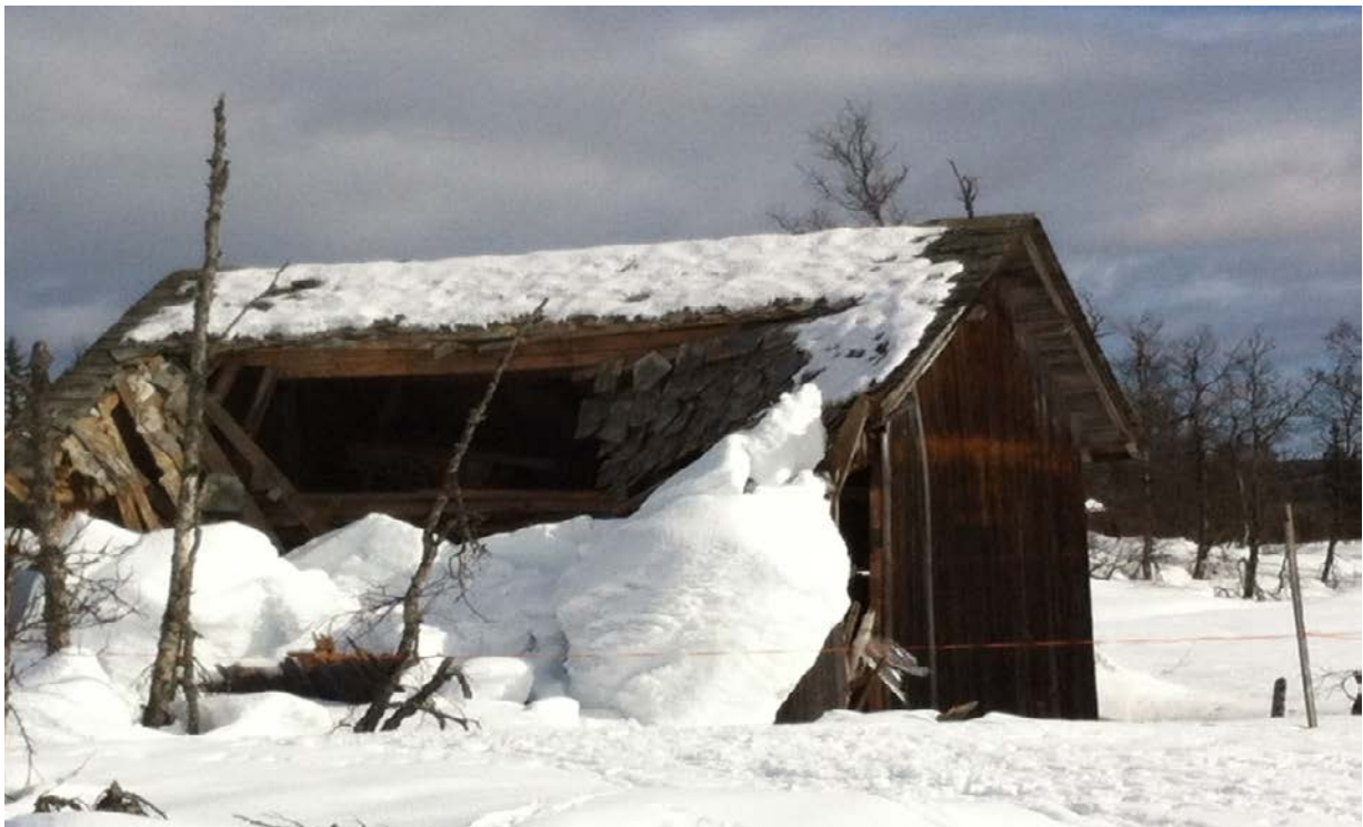
Image 10 The roof of a building has collapsed due to snow load. Oppland, Norway. Photo: NIKU
